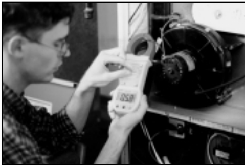
Using a clamp meter to test common loads, such as this heating unit, helps to ensure proper load capacity.
